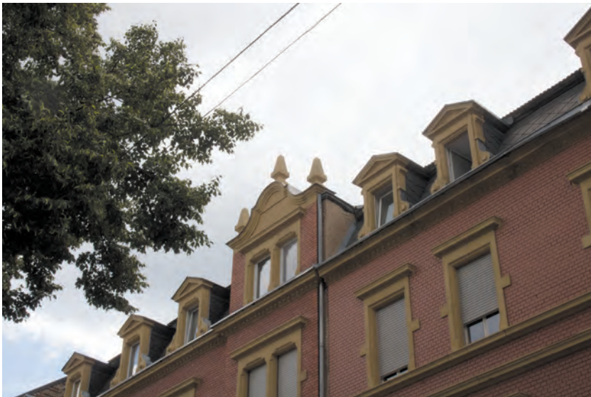
Figure 2. Obelisks on the building in Mainzer Str. 45. Photo by S. and T. Berger
